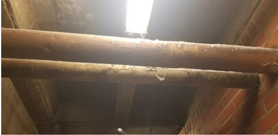
Asbestos-covered pipes located in the basement. Firehouse 23
