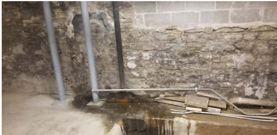
More water leaks into basement
