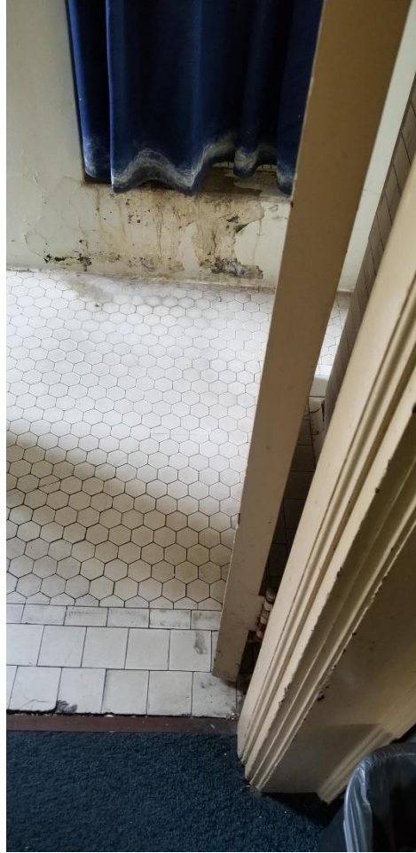
Trim/Mold Issues with shower in Captain's bathroom Firehouse 7
