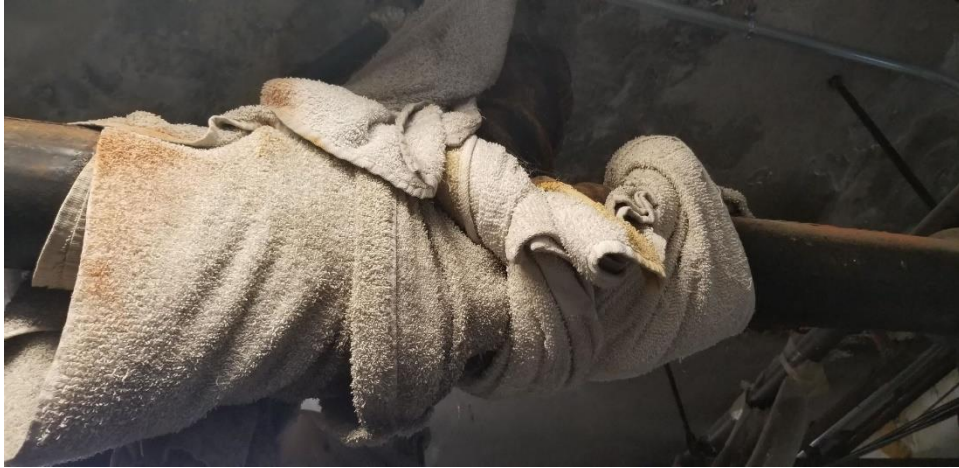
Leaky pipes throughout station Firehouse 17
