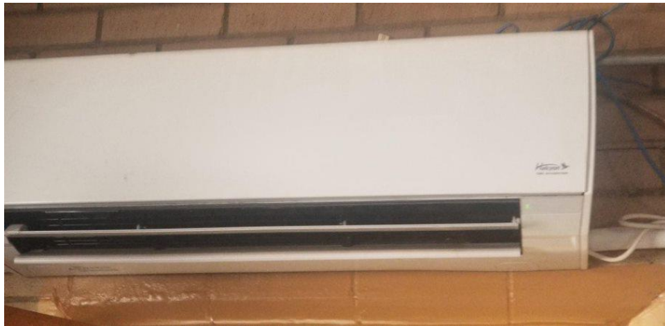
Mini split A/C does not provide enough cooling for the bunkhouse portion of the fire house. Firehouse 24
