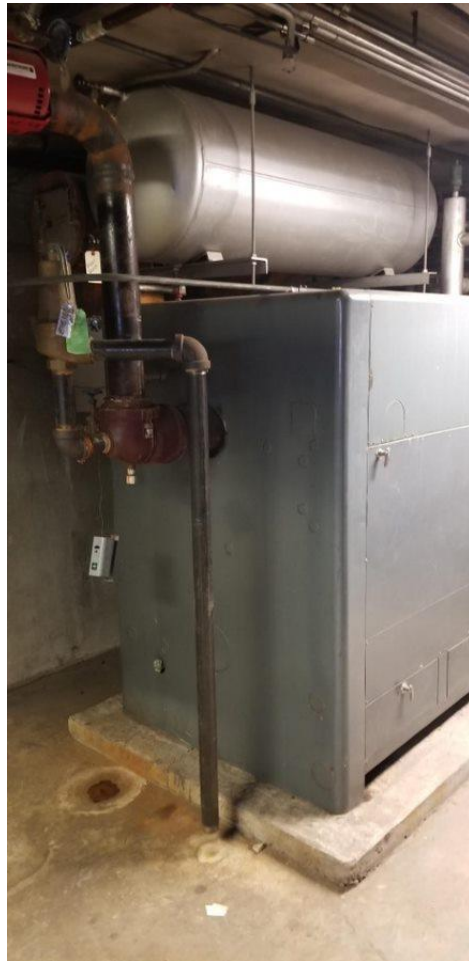
No control over the boiler, so it is either fully on or off, no in-between. Firehouse 24
