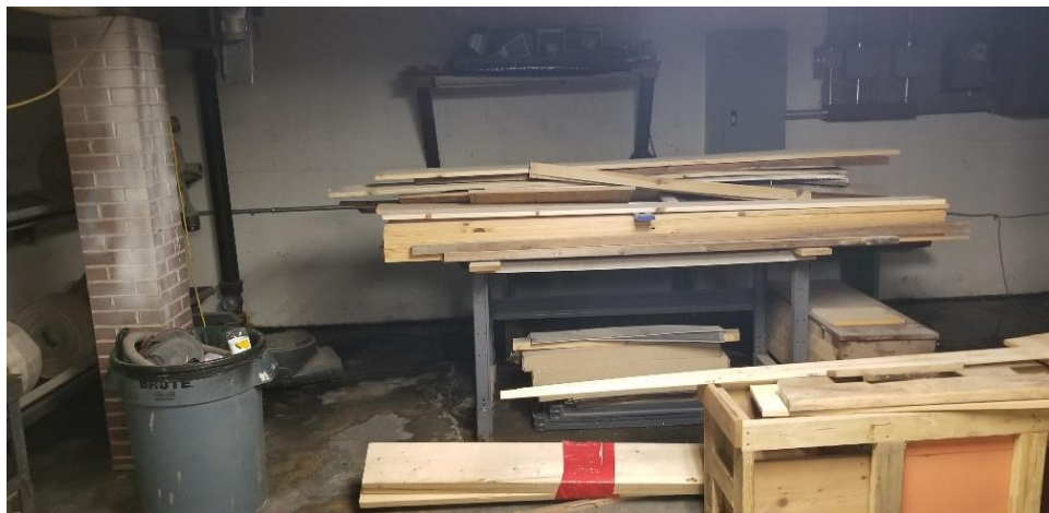
Leaking water into the basement Firehouse 4
