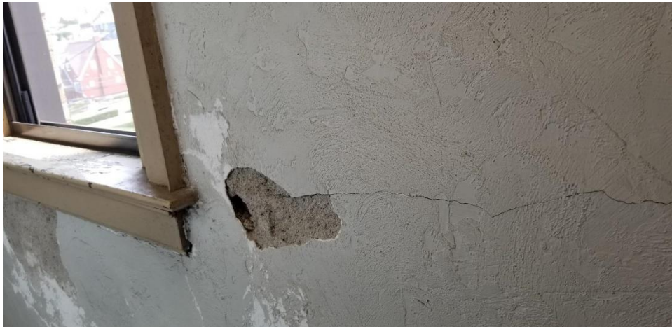
Paint chipping on the walls of the firehouse. Firehouse 7
