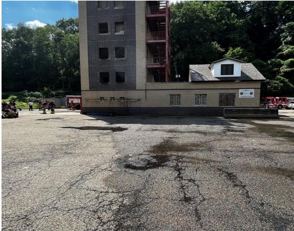
More potholes in the pavement around the practice building Fire Academy
