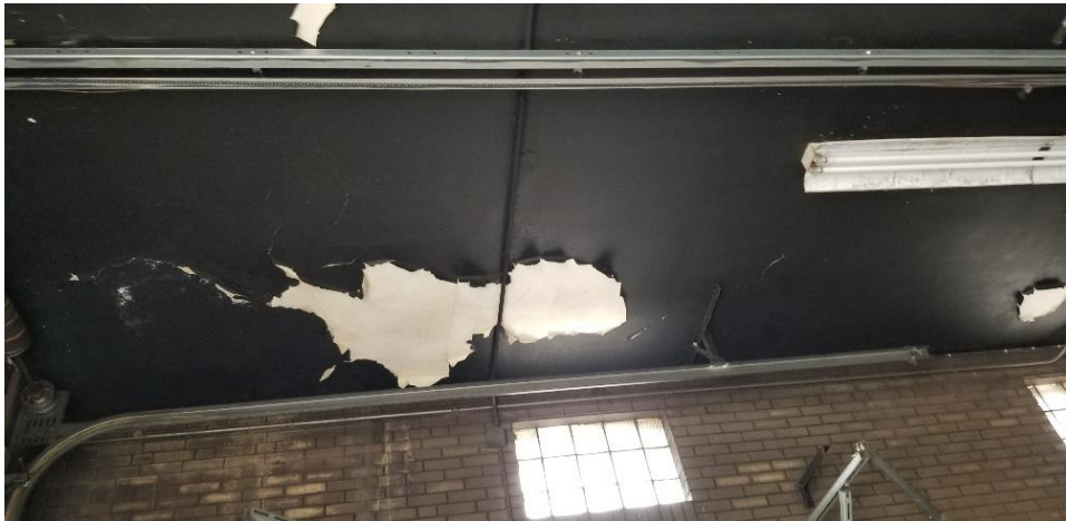
Paint peeling on ceilings Firehouse 4
