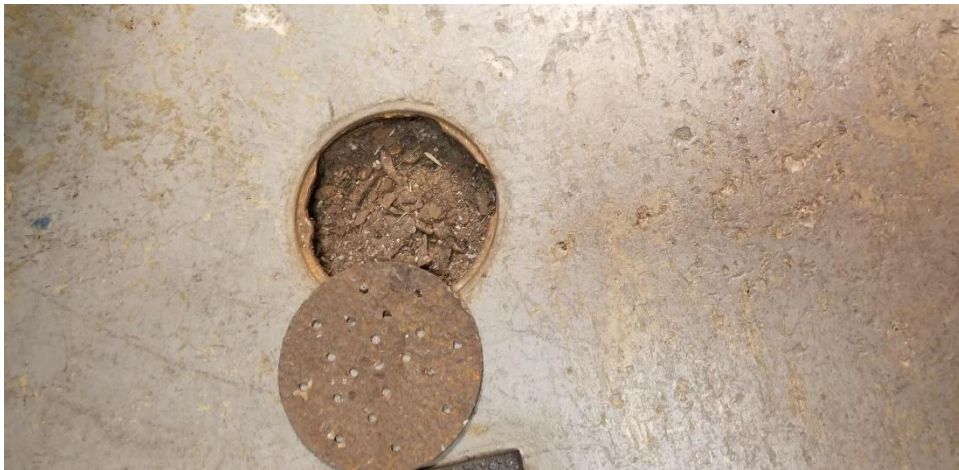
Floor drains are non-flowing Firehouse 17
