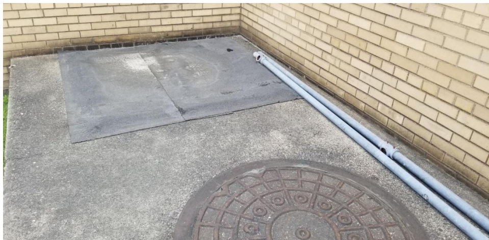
Water drains from the pad into the basement. Firehouse 17
