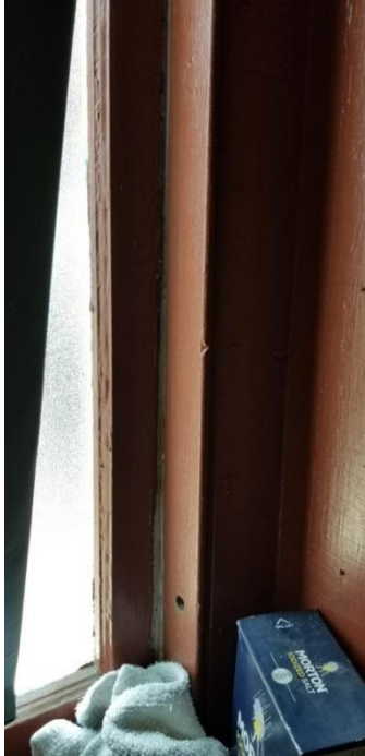
Windows on the 1 st floor were caulked up instead of properly fixed. Firehouse 18
