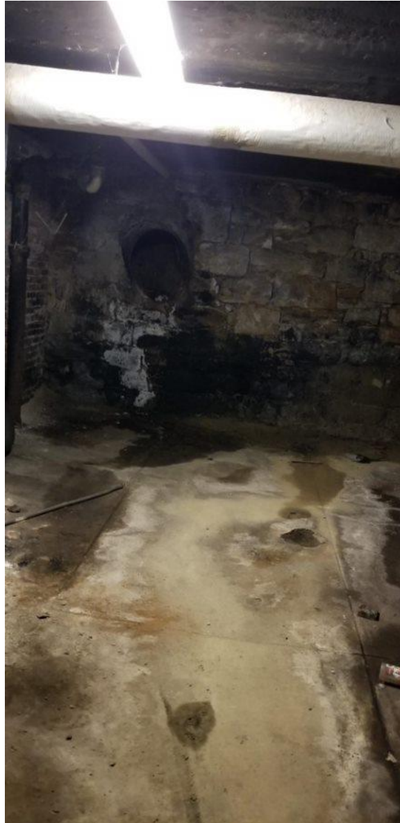
Basement has significant mold issues that limit the amount of time personnel can stay down there, despite being the location of the fire house's washer and dryer. Firehouse 18
