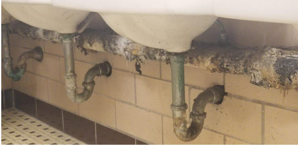
Wraps on plumbing in the bathroom need to be replaced. Firehouse 24
