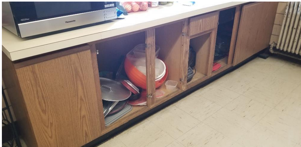
Cabinet doors broken Firehouse 4
