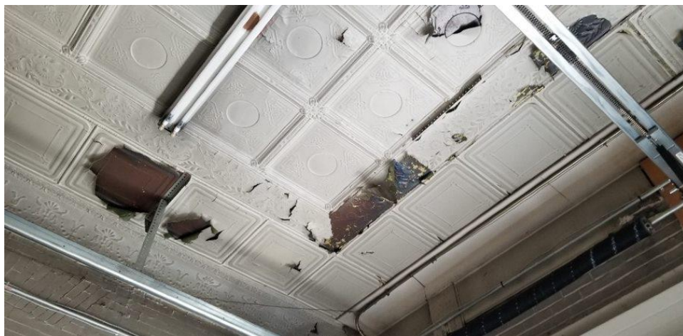
Paint peeling in garage bay Firehouse 35
