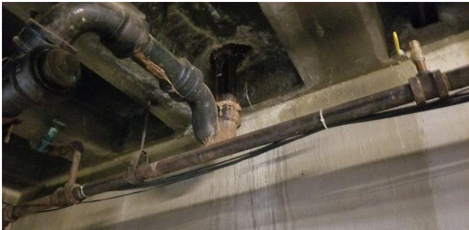
Drain-pipes leak into the basement. Firehouse 23
