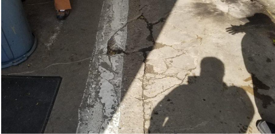
Cracks in garage pad that may have damaged the sewer underneath. Firehouse 18
