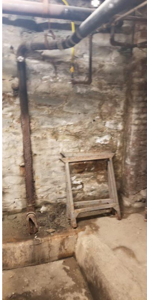
Water leaks into the basement Firehouse 34
