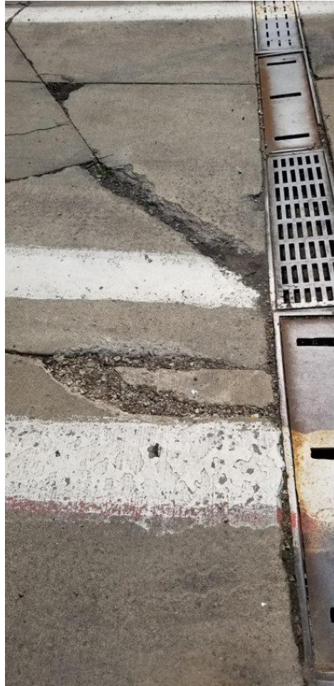
Cracks in driveway pad. Firehouse 17
