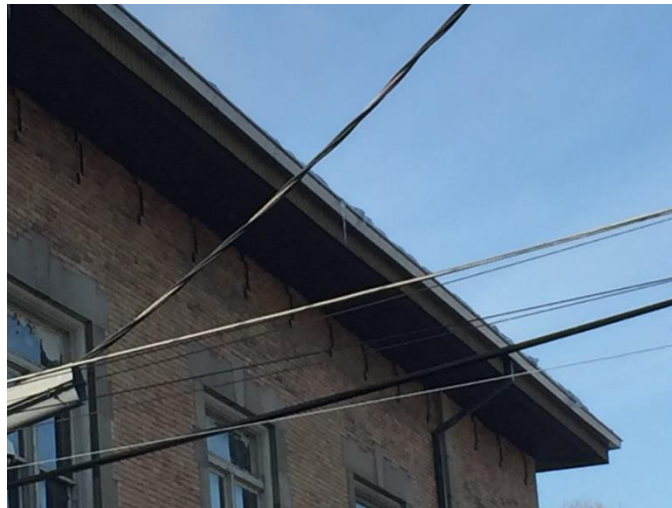
New regular gutters allow dangerous icicles to form, that must be knocked down. Firehouse 18
