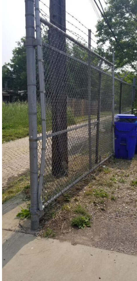
Gate for parking doesn't fully close, allowing trespassers in. Firehouse 17
