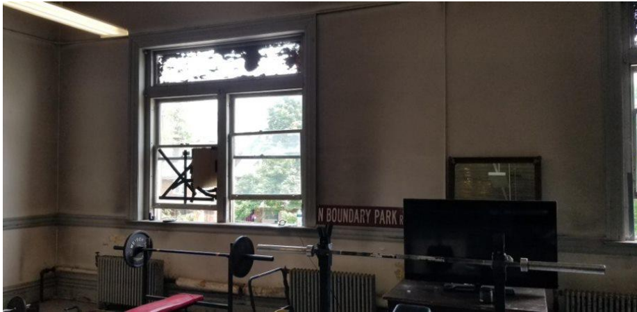
Broken windows on the 2 nd floor that haven't been replaced, allowing significant water leaks. Firehouse 18
