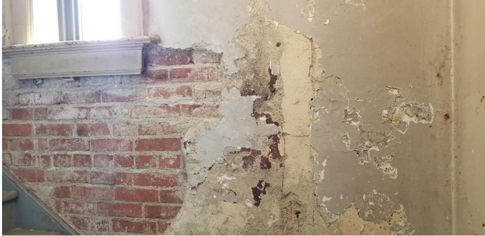
Plaster/Lathe falling off the walls of the stairs. Firehouse 7
