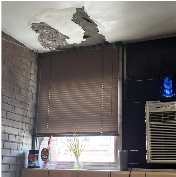
Ceiling Leaks, Kitchen Firehouse 24
