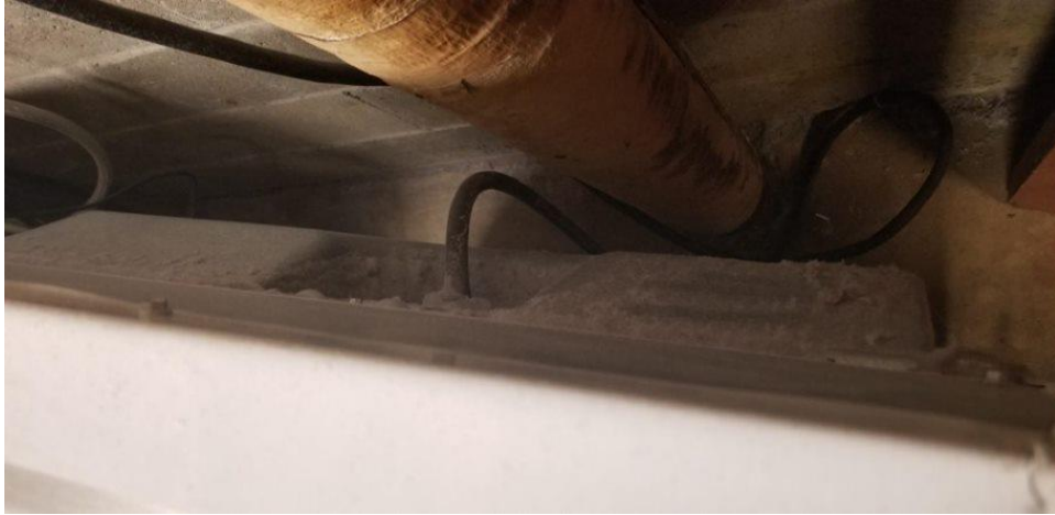
Dryer is not vented, allowing lint to cause significant issues to electronic basement equipment. Firehouse 23
