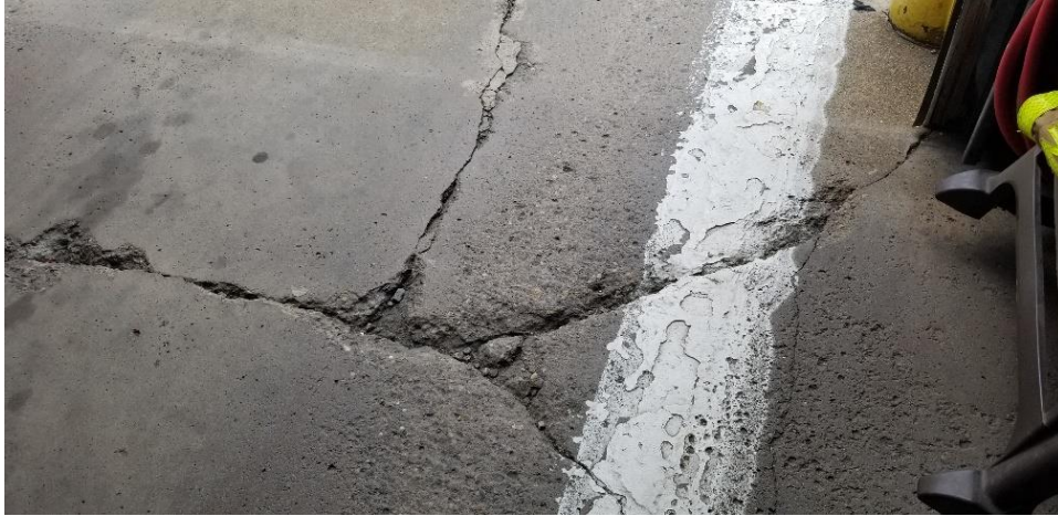
Cracks in the garage pad Firehouse 4
