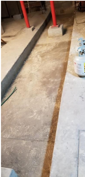
Basement sewer overflows into the trench. Firehouse 7
