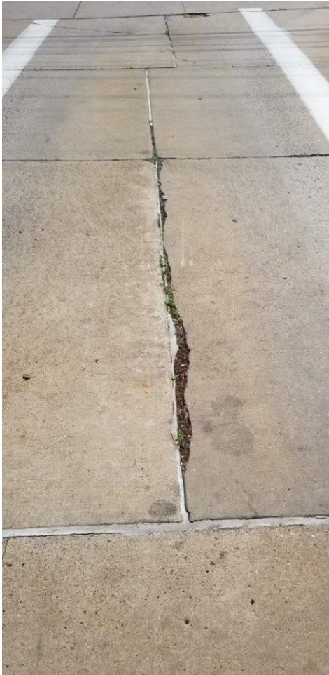
Cracks in the pad Firehouse 23
