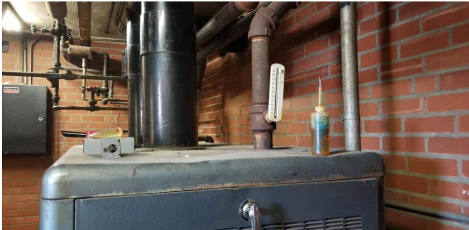
HVAC room smells of gas. Firehouse 23
