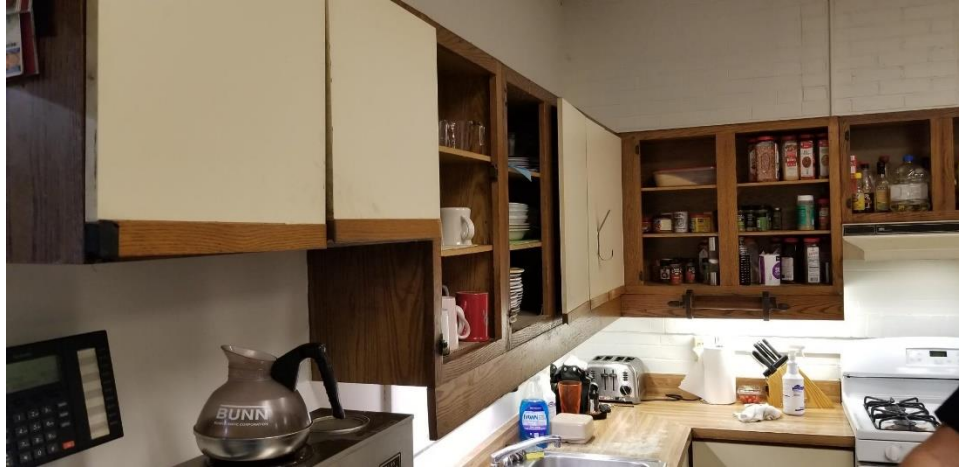
Broken cupboards Firehouse 7
