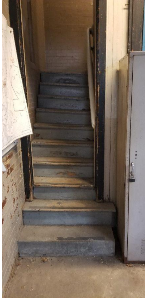
Steps are slanting to one side, which has led to at least one injury resulting in lost time. Firehouse 35
