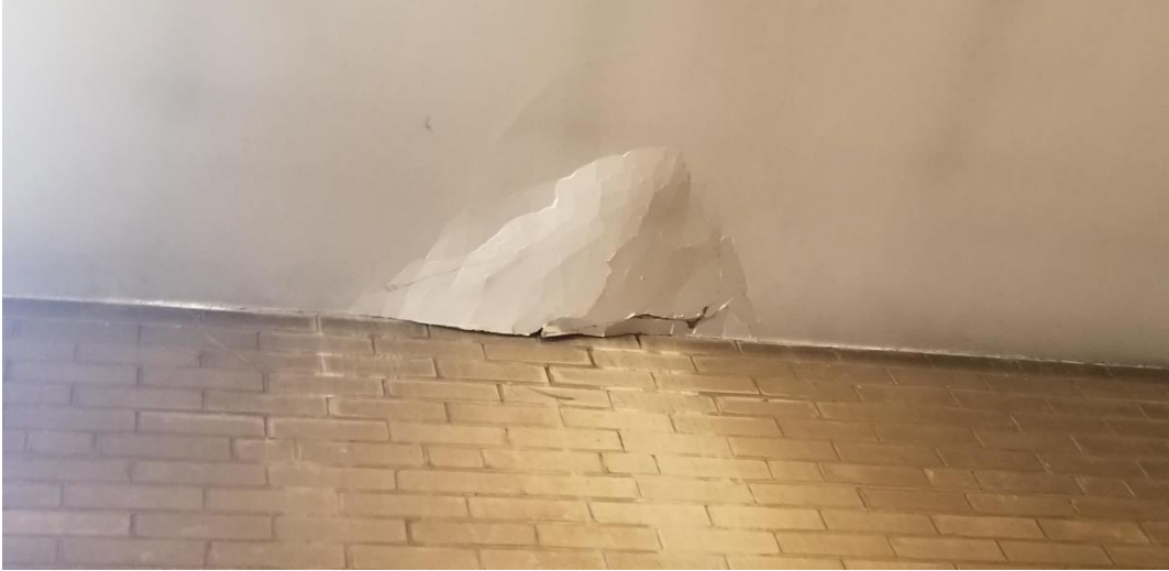
Ceiling Leaks, Garage Bay Firehouse 24
