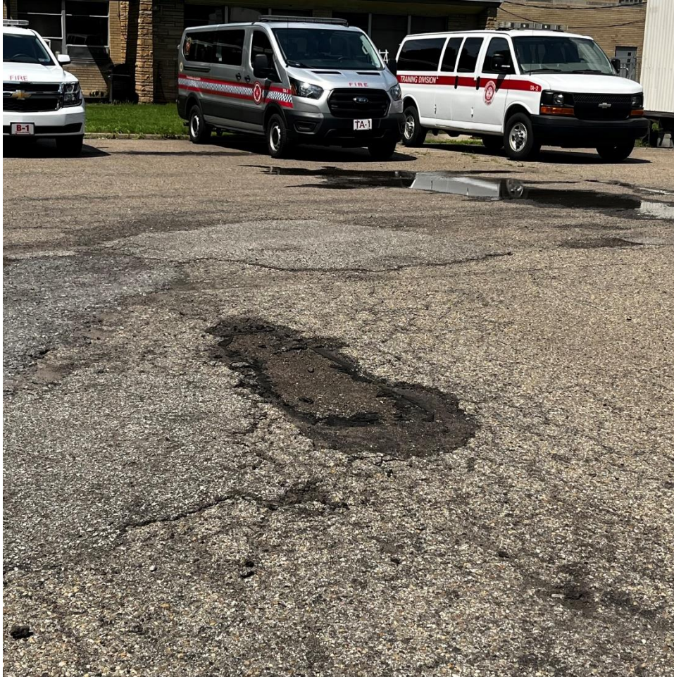
Potholes in the pavement Fire Academy
