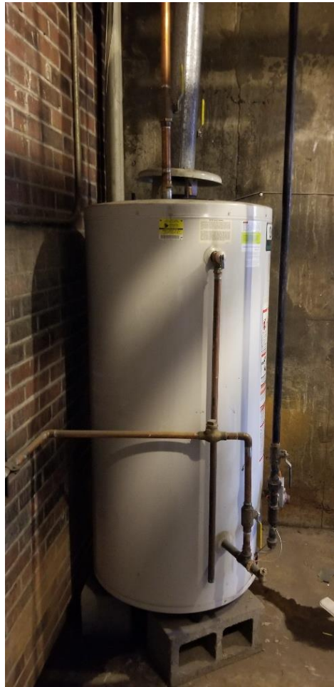
Water leaks onto the furnace and extinguishes the pilot flame on the boiler, leaving the station without hot water Firehouse 4
