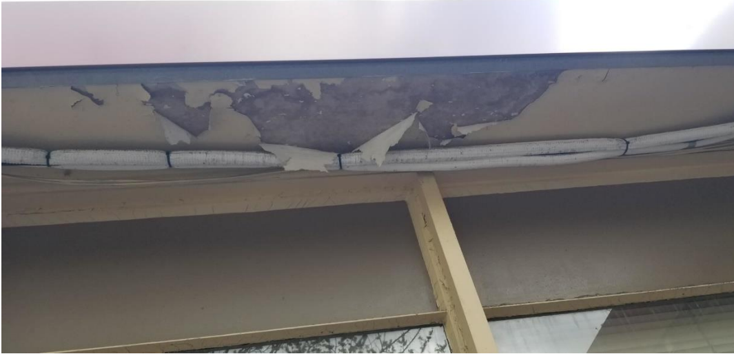
Over time, roof leakage or masonry damage from clogged gutters has damaged portions of the ceiling. Firehouse 24
