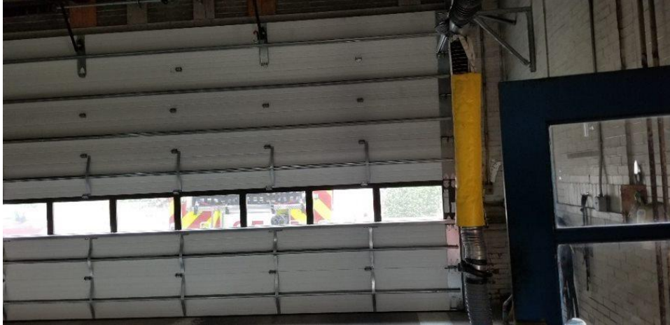
Station door was not working at the time of the auditors' visit. Firehouse 35
