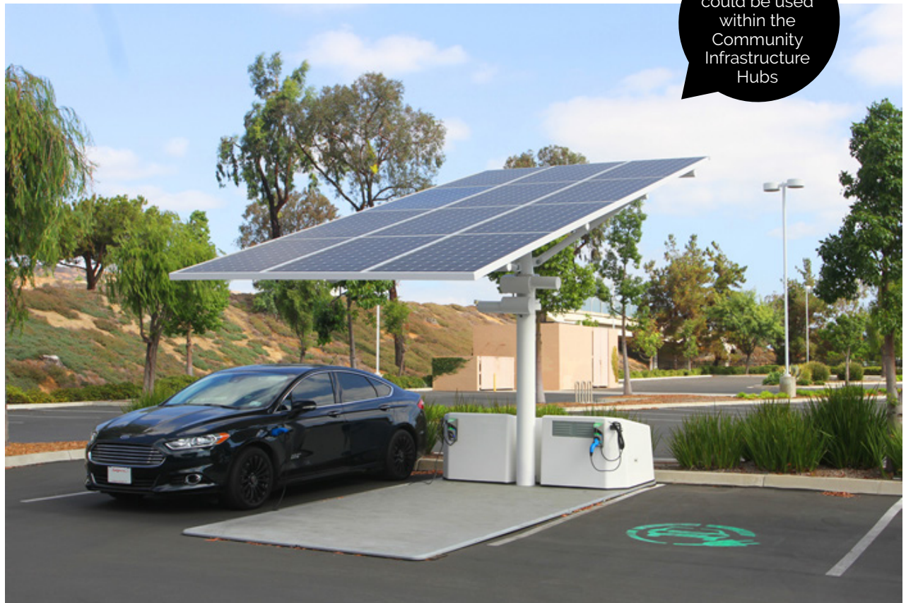
EXAMPLE OF ELECTRIC VEHICLE CHARGING STATION POWERED BY SOLAR PANELS
