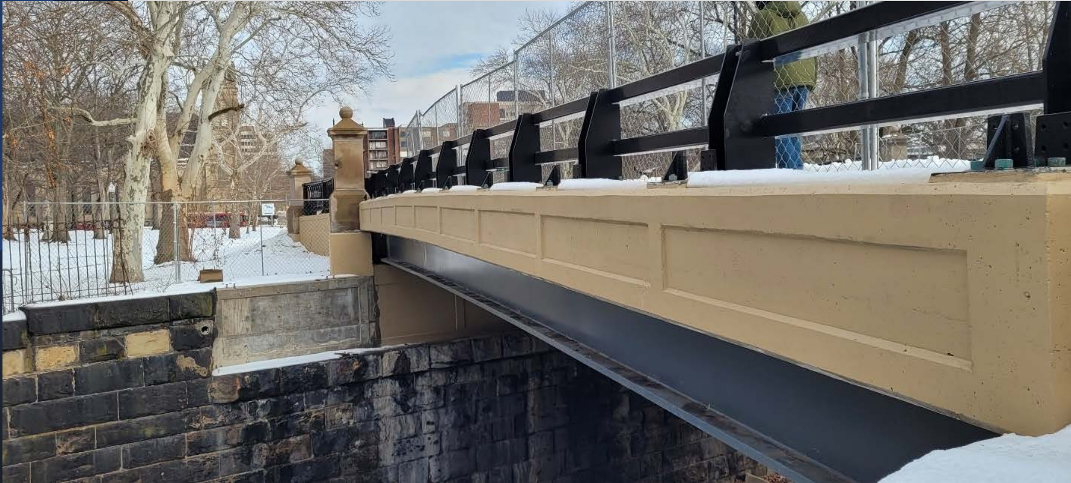
Detail of concrete panel and steel girder colors used on the W. Ohio Street Bridge.
